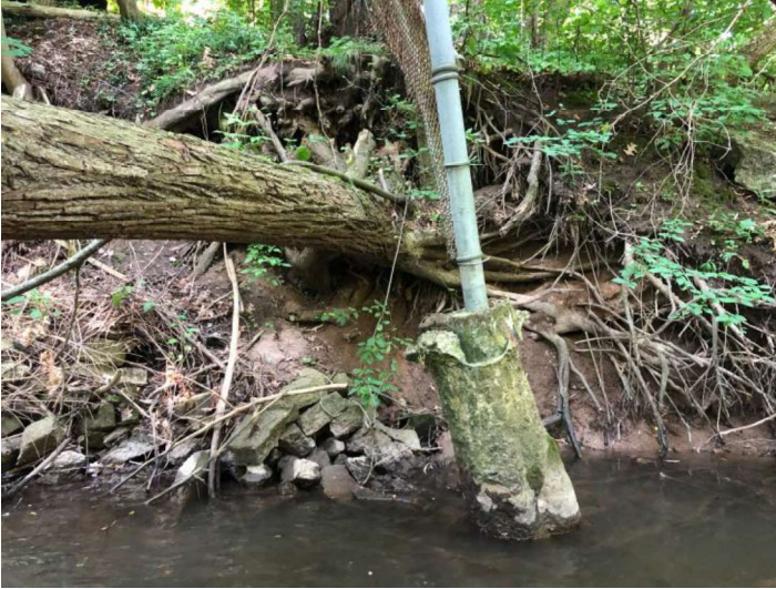
Photo 1: Erosion of property line fence directly downstream of outlet channel tie-in.
